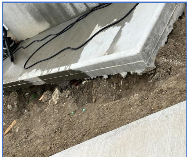
Clay voids under concrete structure and undefined swale
